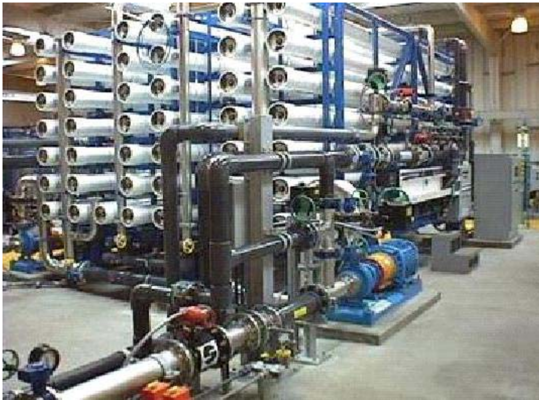
The Nanofiltration Train at Port Hueneme Brackish Water Reclamation Demonstration Facility
